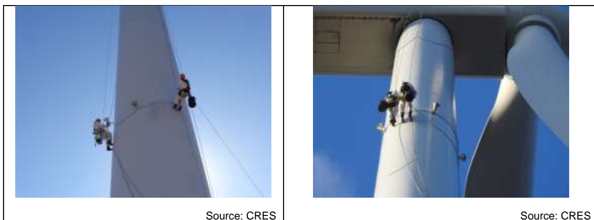
Figure 7. (a), (b) Views of the installation of HD video surveillance system at the wind turbine in North Greece.
