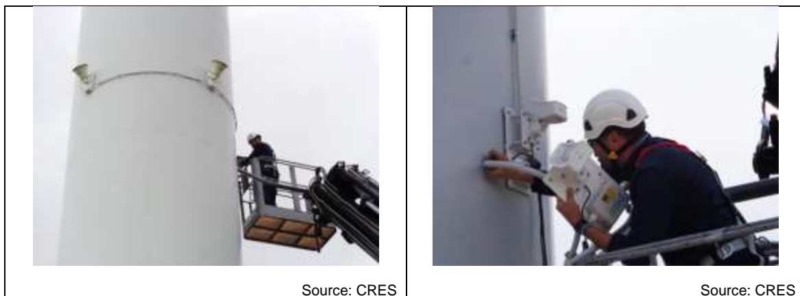
Figure 6. (a), (b) Views from the installation of the video surveillance system at CRES Demonstration Wind Farm-PENA.
